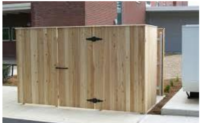
Example of mechanical enclosure
