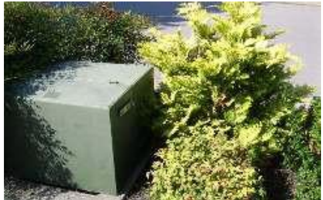
Utility connection screened with plantings
