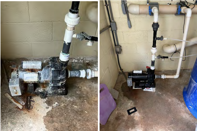
Pool Chlorine Pump
