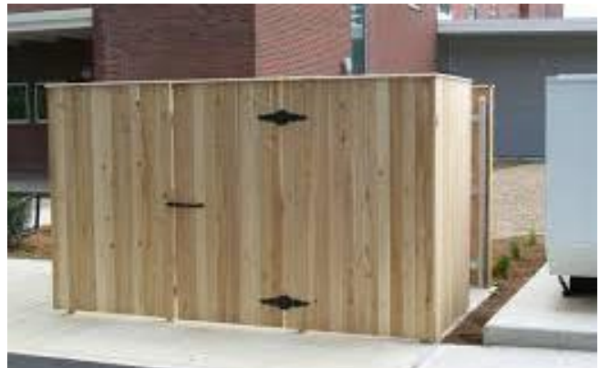
Example of mechanical enclosure
